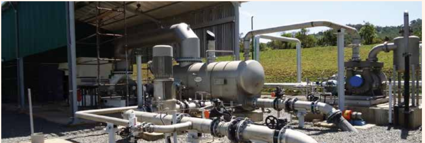
Eburru Wellhead Geothermal Power Plant.
