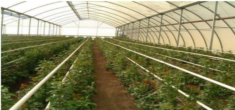
Pipes carrying geothermal brine in Oserian Flower Farm Greenhouse
