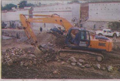
Upgrading of Thika Highway is one of the projects being funded by the African Development Bank. The superhighway is set for completion next year.
