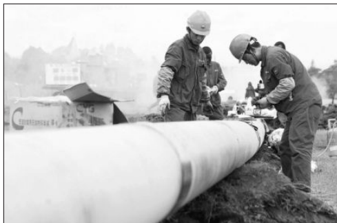
Workers put final touches on the Western Kenya pipeline. A consortium of local banks funded the project to the tune of $83bn.
