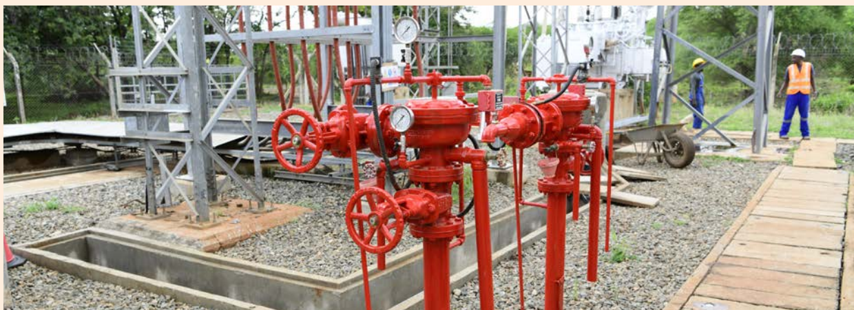
▲ Fire Risk Mitigation at Gitaru Station
