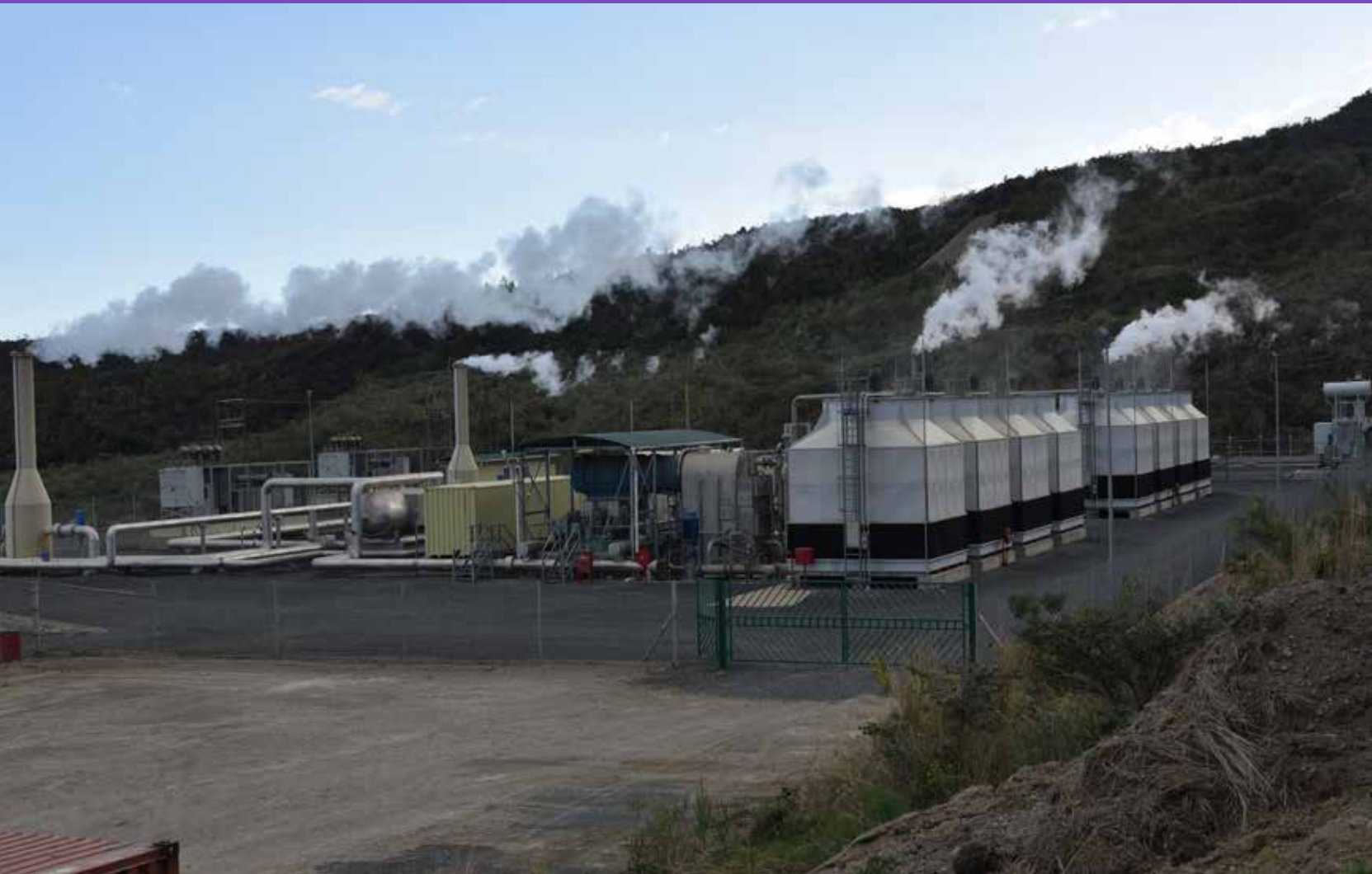
Olkaria Wellhead Plant
