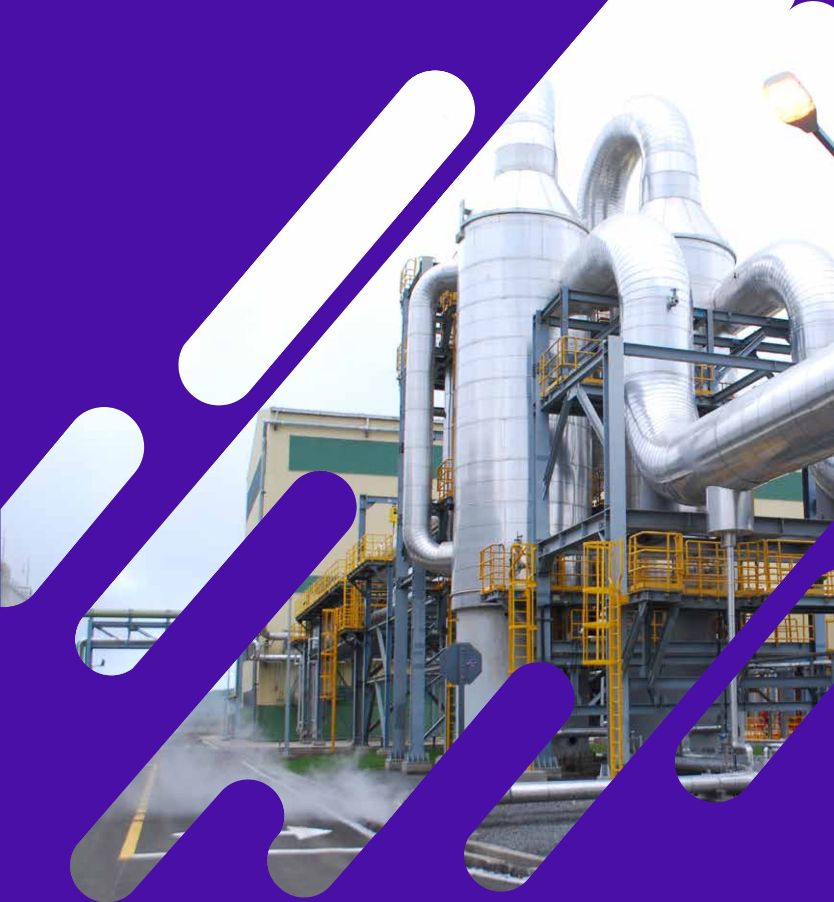
Olkaria IV Geothermal Power Plant
