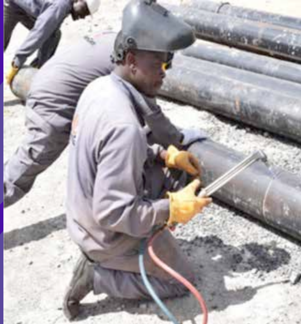
KenGen Olkaria Team undertaking the 1st ever in-house steam pipe design, set up and successful commissioning
