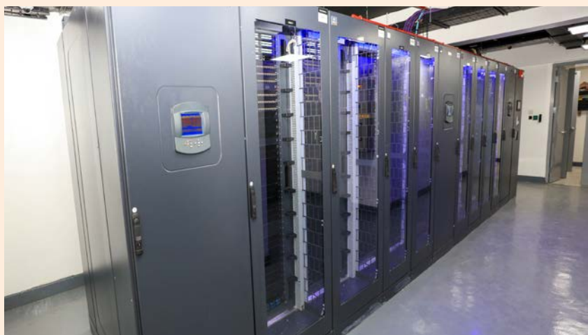
KenGen Data Centre
